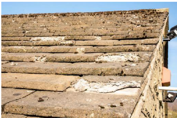
CRUMBLING EXISTING ROOF TILES
